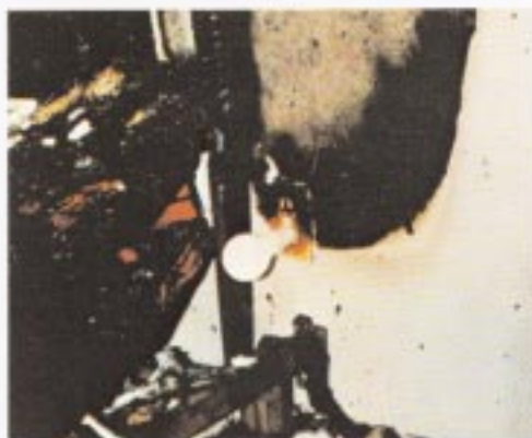
① This wall receptacle in the apartment master bedroom shows the extent of fire damage to bed frame, wall and outlet plate, while circuit operation is demonstrated by light. Recorded room temperatures are shown in Graph A. See Diagram II.
