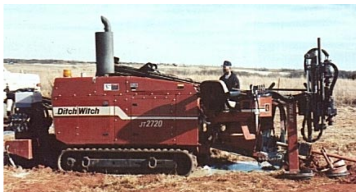
At Left: In the foreground is the reamer attached to the drill string. Barely visible from 1,000 feet on the horizon is the drilling machine. Above Right: A close-up look at the powerful Ditch Witch ® JT2720 that quickly and easily pulled in the 1,000 ft. string of Bore-Gard.
