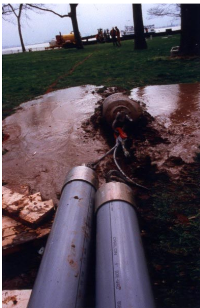
Left: Using a 16" backreamer, two 6 inch Bore-Gard ducts are being pulled into the 190 ft. bore
