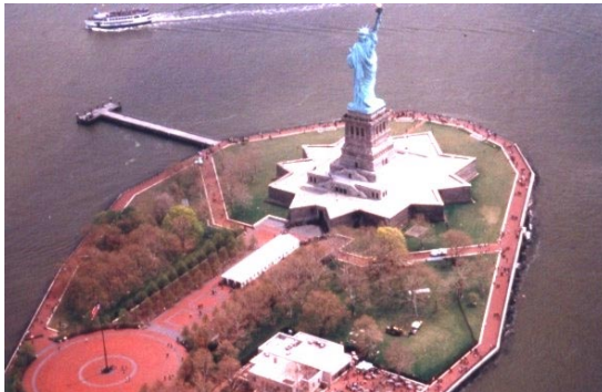
Left: Limited spaces and minimizing disruption to the pristine environment and daily tourist activities made Horizontal Directional Drilling and Carlon Bore-Gard the ideal solution.
