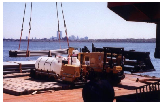
Above: Bore-Gard was transported to the island, after visiting hours, on a 10,000 s. ft barge pushed by a tugboat.
